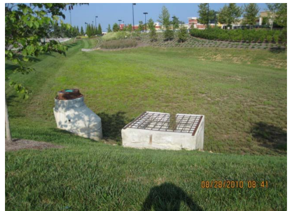
Figure 7. Landscaped and well-maintained permanent stormwater detention pond.
