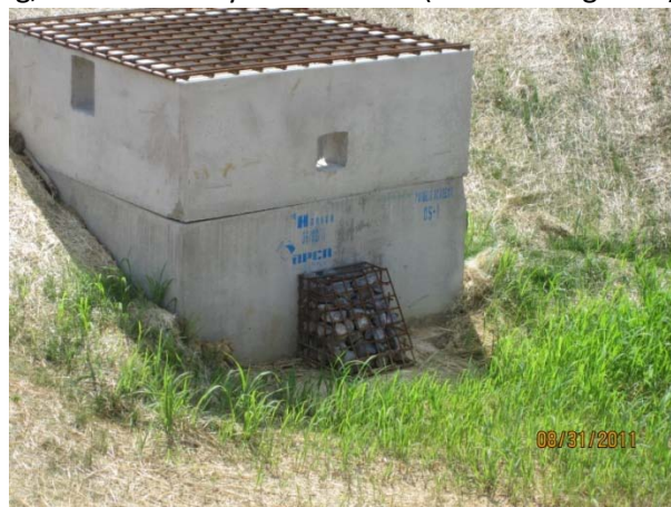
Figure 2. Unacceptable hole & sediment filter arrangement at bottom of riser and sediment pond.
