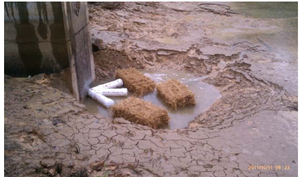
Figure 8 illustrates a condition where a sediment basin was converted to a detention pond without removing the accumulated sediment. Figure 8. Former sediment basin converted to a stormwater detention pond without removing sediment.
